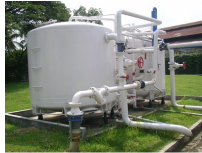
Evaluation of process water treatment
