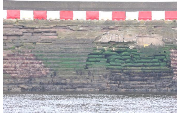
Figure 3 – Damage to Southern Stone Face
